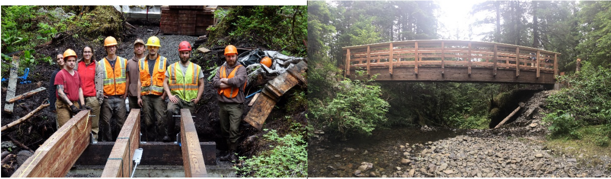
2017 Trail Mix Crew and final bridge installation on Treadwell Ditch at Paris Creek
